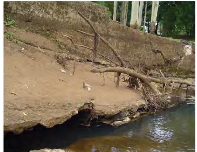
Plate 11 - Undercutting of the apron on the upstream side of the weir
