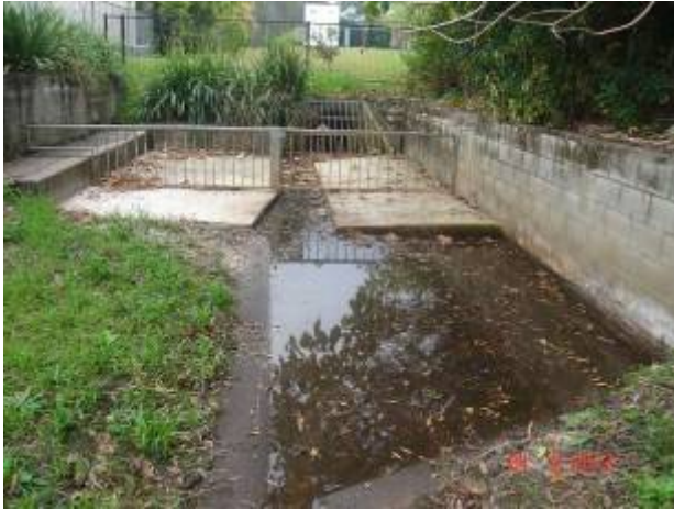
Photo 3 – inlet area showing water ponding following 1 st rain event after dry period (24/9/12)
