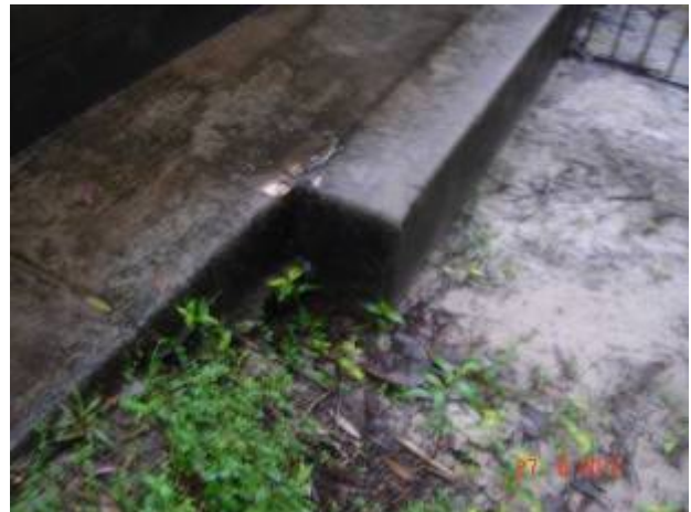
Photo 12 – exposed footing of upper retaining wall (13/9/12)
