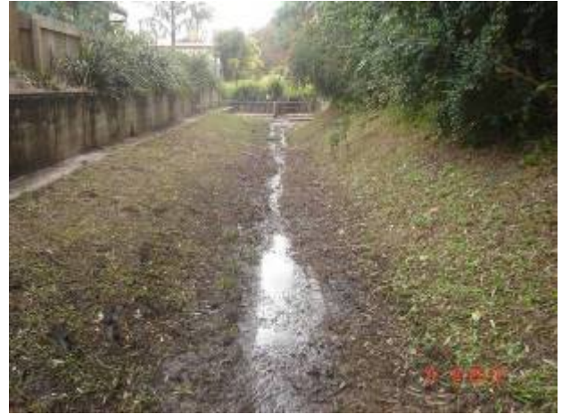
Photo 4 – v-drain showing silt build up and water ponding (9/8/12)
