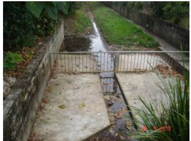
Photo 6 – inlet area and v-drain following 1 st rain event after dry period (24/9/12)
