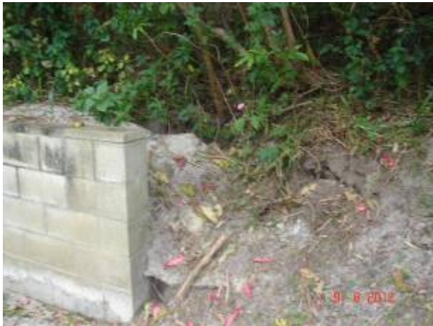
Photo 9 – erosion at end of retaining wall at inlet area (9/8/12)
