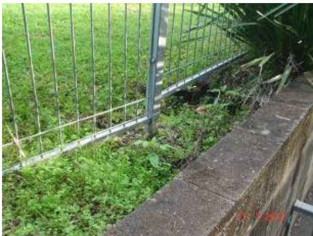
Photo 13 – area of subsidence behind retaining wall (17/7/12)
