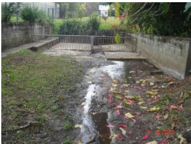
Photo 1 – inlet area and v-drain showing silt build up and water ponding (9/8/12)
