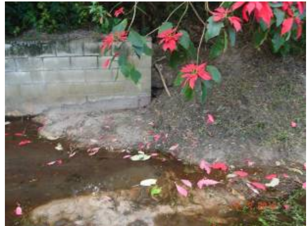
Photo 10 – silt from erosion in concrete inlet area (17/7/12)
