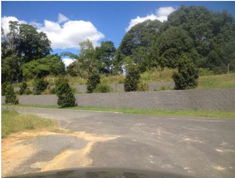
Figure 5 - Existing two tier retaining wall near southern boundary (adjacent to shelter belt)
