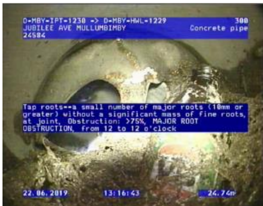
Major root intrusion obstruction
