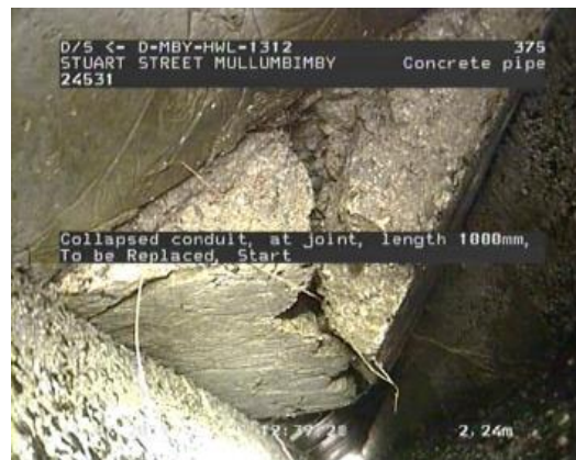
Roof of stormwater urban main collapsing
