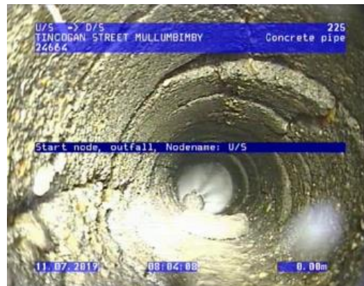
Major cracking and radial deformation
