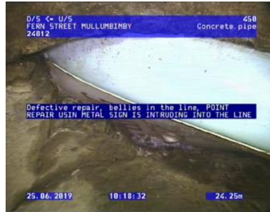
Defective repair with a street sign
