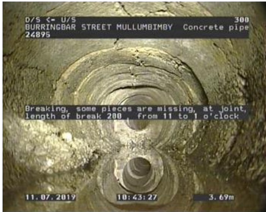
Major cracking and radial deformation
