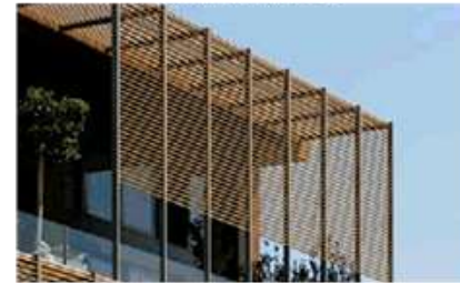
Solar Shading to reduce summer heat.
