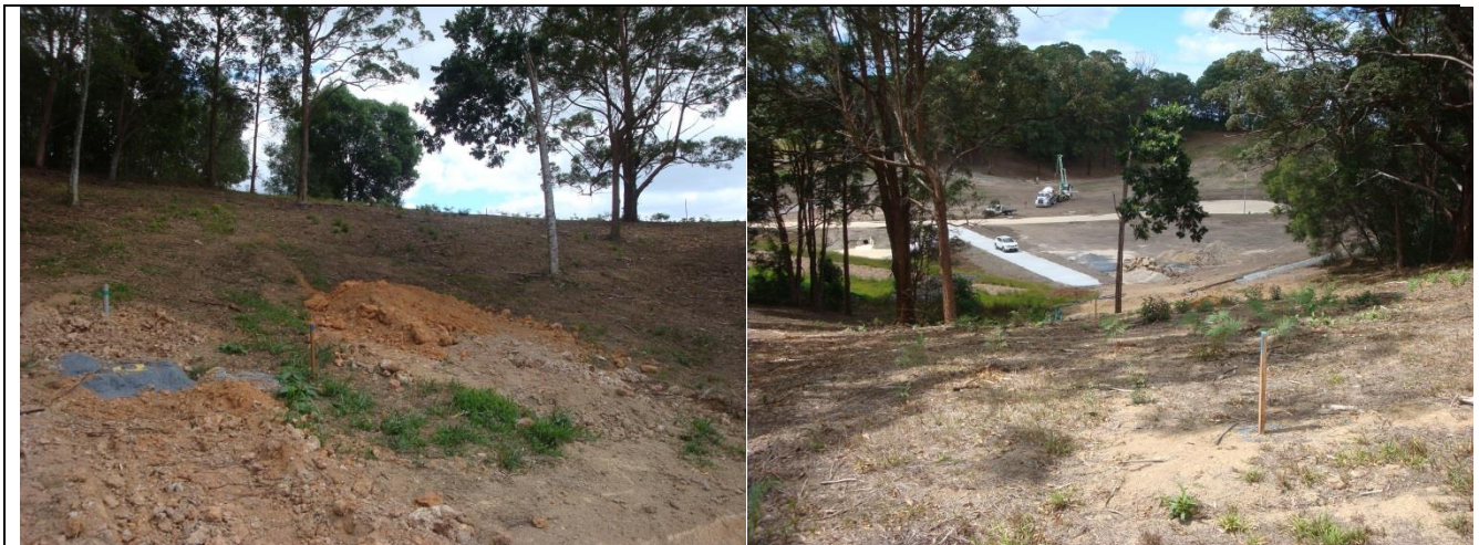
Photo 1 – Proposed path of stormwater pipe (water pipe inspection port in left foreground of photo)
