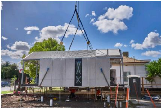
First transportable housing unit is craned onto site in Melbourne's inner west.
