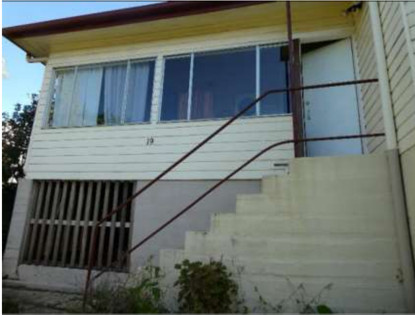
Front entrance as existing; Front sunroom to be converted back into verandah/deck.
