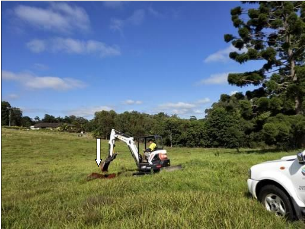
Photo 4 View SW showing gentle sloping land towards a gully, BH2 location at arrow.
