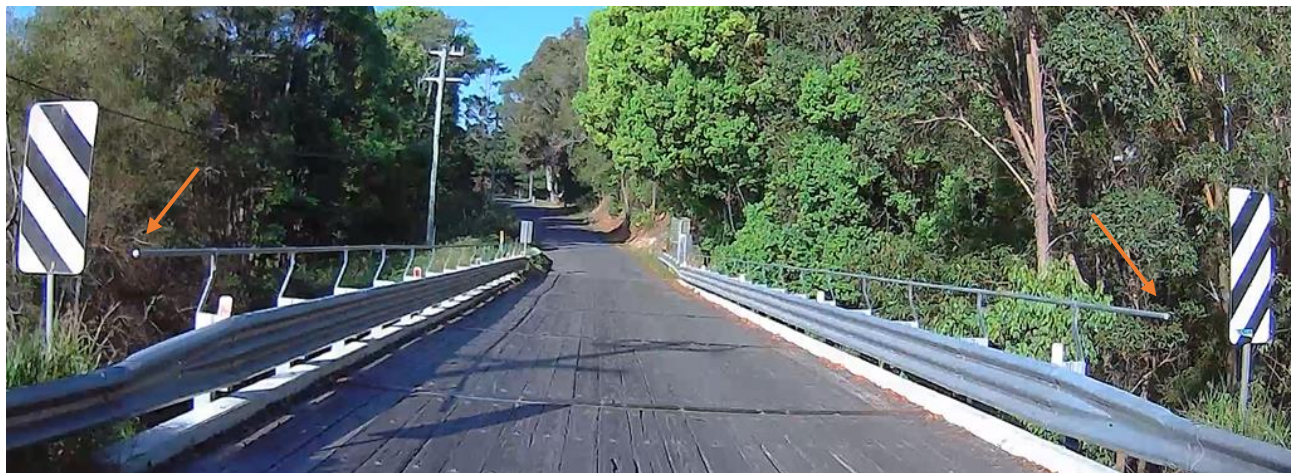
Photo 20: Potential spear hazard?
