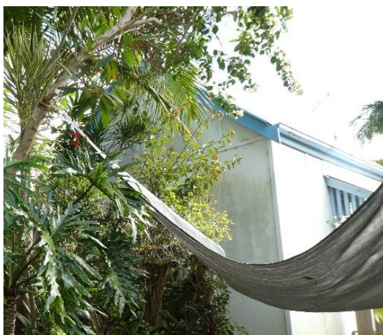
40 The Terrace – Camouflaged by vegetation this is an early 20 th century cottage with high pitched roof and projecting gable element which has been over clad in fibre cement.
