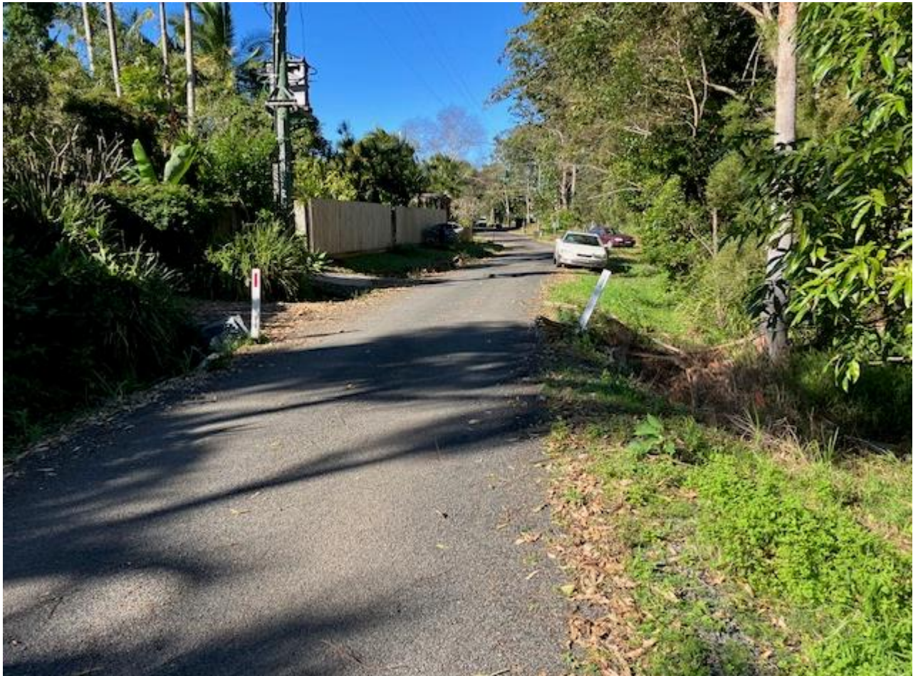
Image 7: spoon drain along the east side of road (left in photo) with culverts running under driveways and road, channelling the water to the west side of the road
