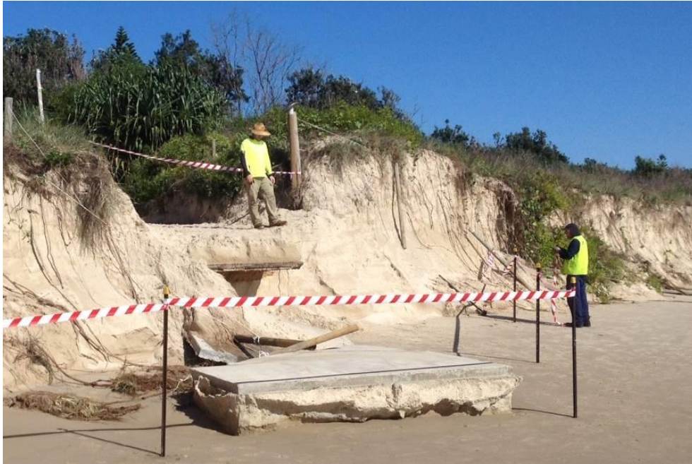
Figure 2. Damaged section of access path (source: BSC)
