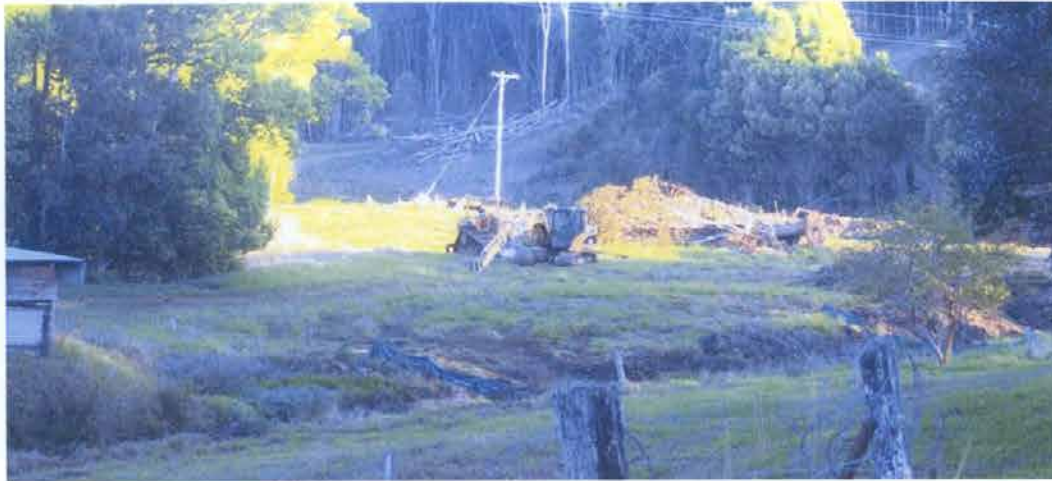
Picture C. Ineffective silt traps.
