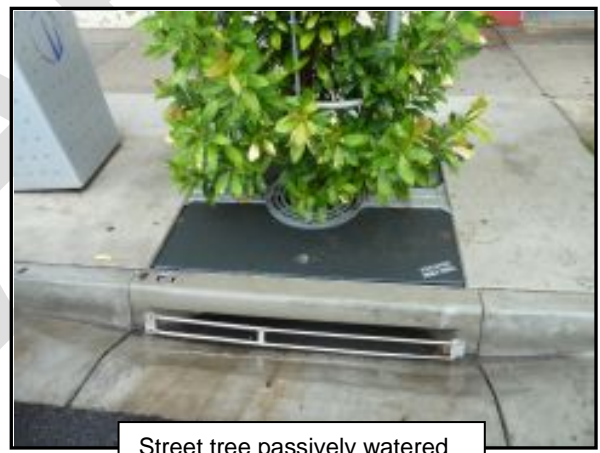
Street tree passively watered from stormwater runoff
