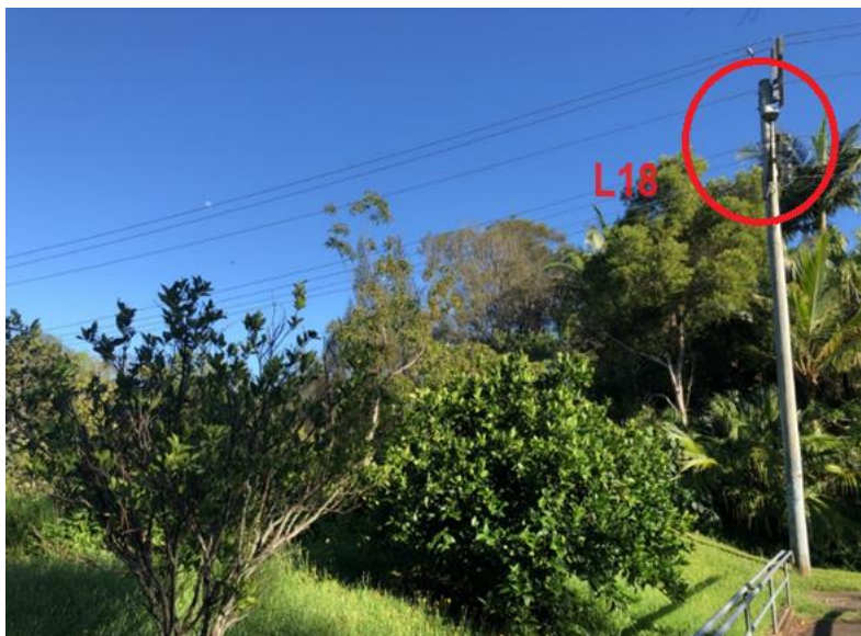
Plate 17: Essential Energy pole-mounted streetlight at the Helen Street footbridge over Yelgun Creek. There are few other streetlights in proximity to the creek. Some vegetation provides light screening between the creek and this light source. The direction (downfacing) and low wattage (18W) would provide low level illumination to the waterway and adjacent vegetation. Replacement of this light with a low-level bollard could be considered.
