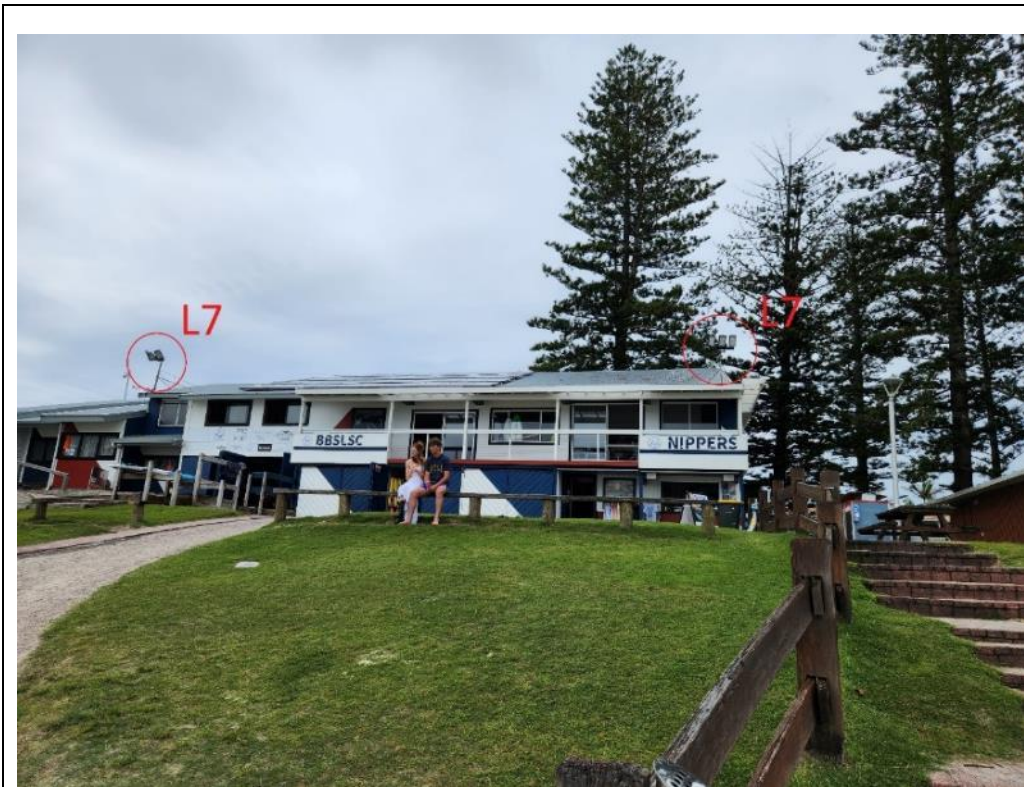
Plate 6: Roof mounted floodlights directed towards the beach at the Byron Bay Surf Life Saving Club (L7).
