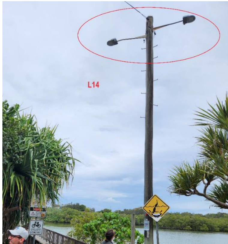
Plate 13: Double light fitting with problematic light spill (L14) immediately adjacent to Simpsons Creek.
