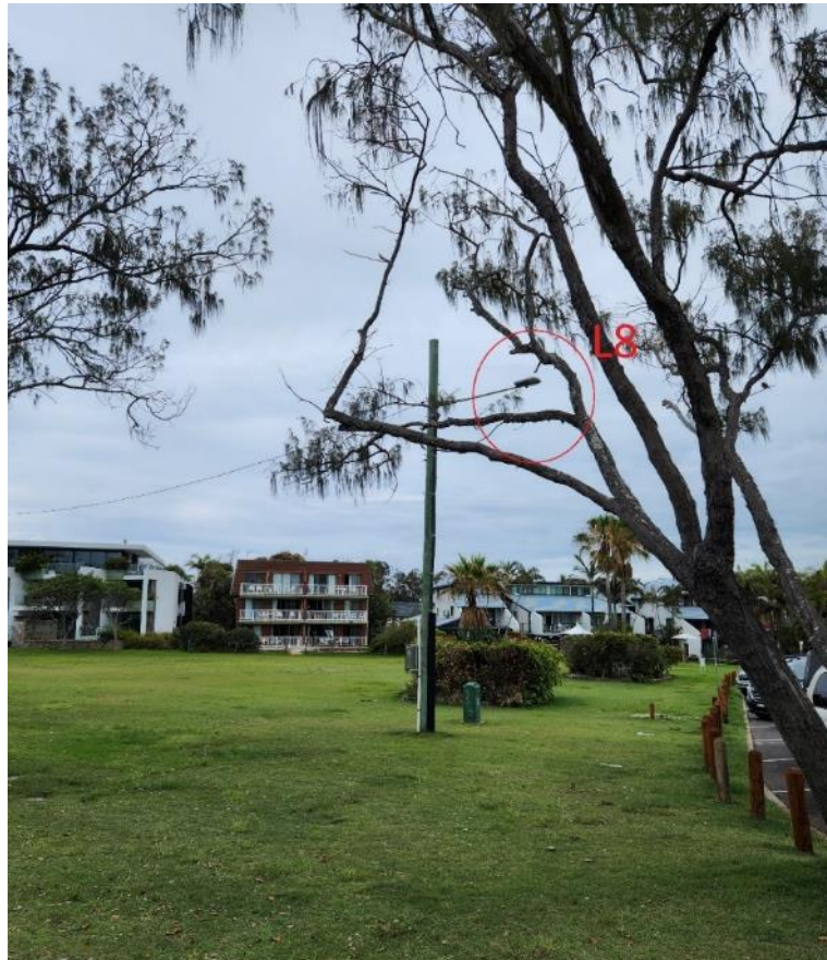
Plate 7: Essential Energy road light fixtures located in grassed area, distanced from intended purpose (L8).
