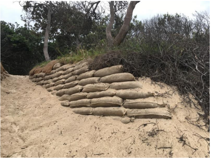
Photo 6: RHS of track – sandbags installed (13/02/18)
