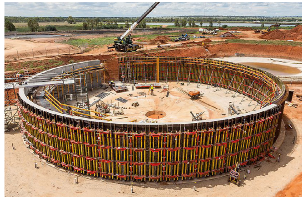
Dubbo Regional Council recently completed upgrades to its STP in order to keep up with expected population growth. Pictured, is one of the two clarifiers included in the upgrade.
