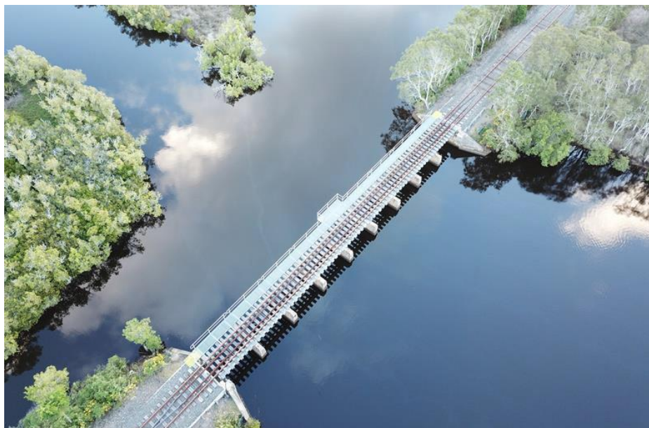
Figure A12.1: Belongil Creek Railway Bridge after restoration by Byron Bay Railway Company
