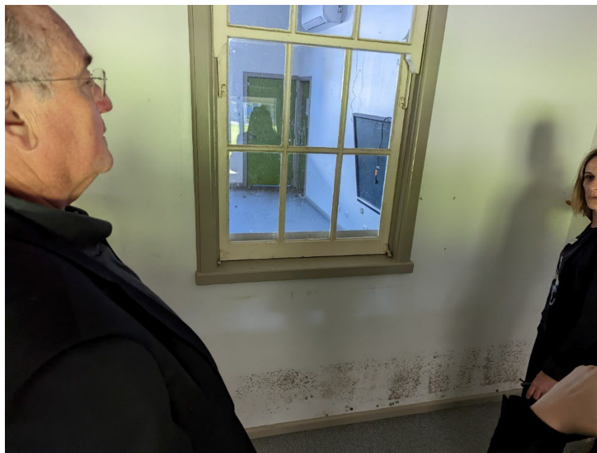
Figure 11 Committee members inspecting mould in affected classrooms at Condong Public School
