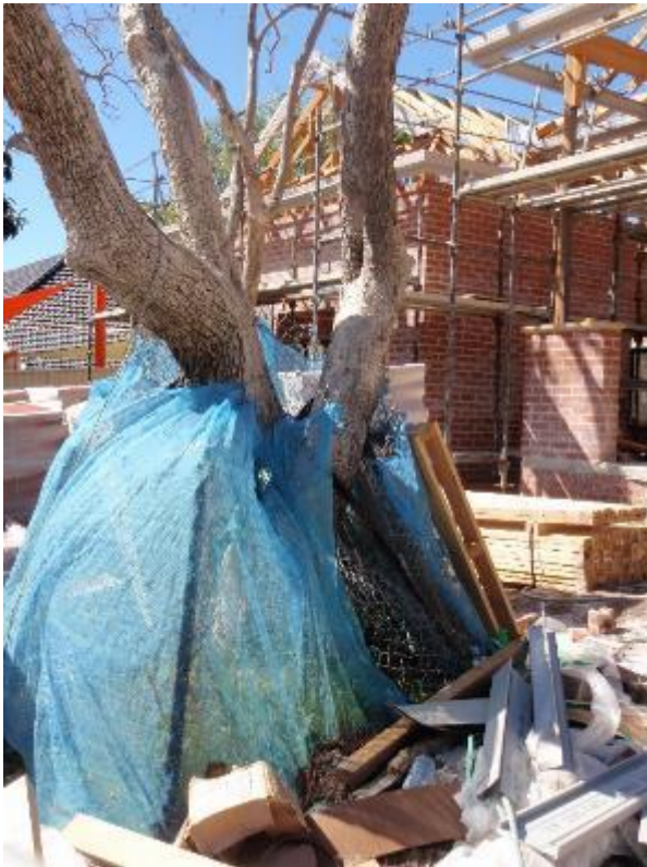
Image 3: Bad – Stockpiling in the TPZ
